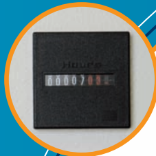
Elapsed time-meter for hepa filter
